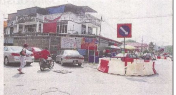
Uncompleted works in Jalan 1/10 and cars parked by the side of the small road make it hard for motorists to manoeuvre safely.
